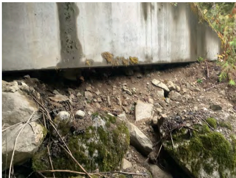
Downstream left fill loss beneath ballast wall
