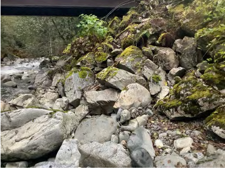
Upstream right riprap scour
